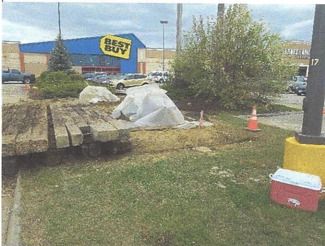
Fig 3. Timber matting con't. Concrete footings for structures E194-10 and F1070134, viewing north.
